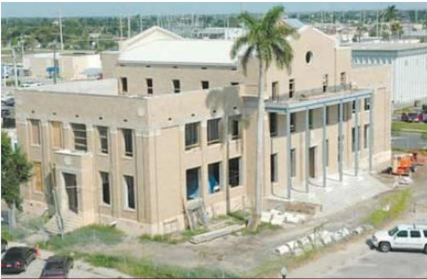
The roof of the Sunloft Center offers a great view of the rapid restoration of the old courthouse across Taylor Street.
