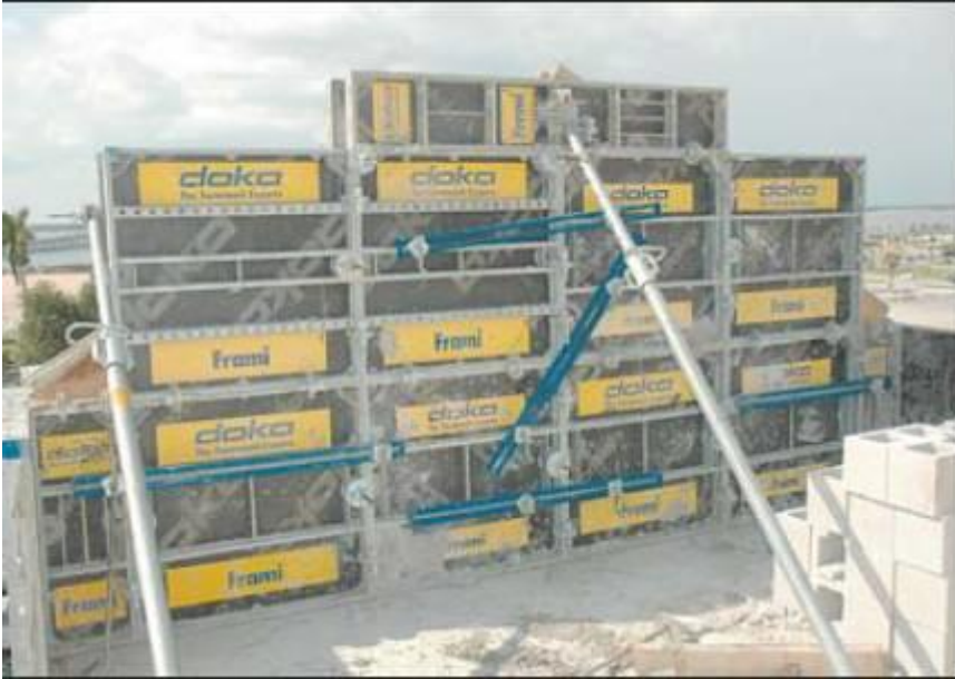
The facade elements along the roof line are made of formed concrete with rebar.
