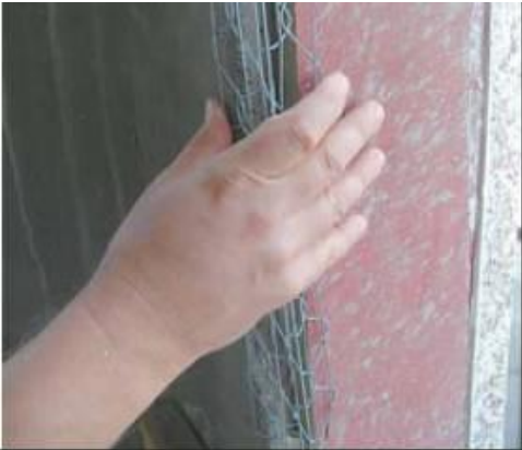
Left, Pantsari holds one of the expensive corner beads, just seen peeking out of the unfinished corner in the top photo and necessary for a perfectly crafted tabby corner like this one in the photo below.
